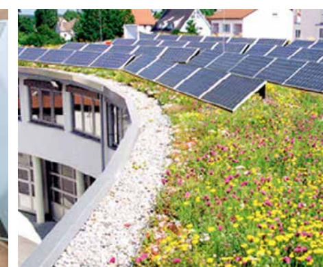
Figure CC.82. Solar Photovoltaic Panels
