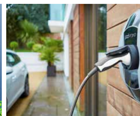
Figure CC.81. EV charging point at home
