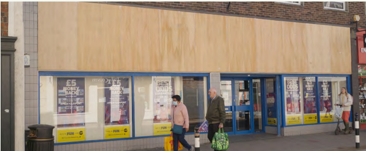
A poor example of an excessive fascia that takes up about 50 per cent of the entire shopfront. This dominates and makes the shop look like a billboard rather than a commercial premises
